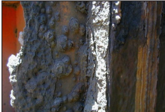
Failed paint system after 1 year exposure
