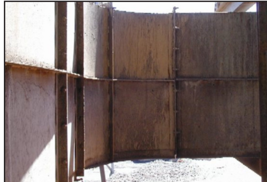
ARC S1PW applied to exteriors of ductwork
